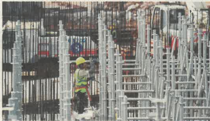
Work is in full swing at the construction site of the Nanningbei railway station in Nanning, Guangxi Zhuang autonomous region. Photo: Xinhua
